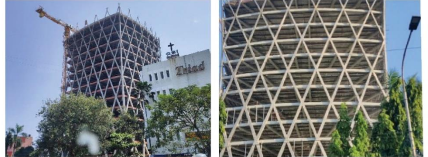
Outer Support Structures
